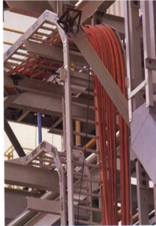
Pacific Composites' FRP cable ladder being installed in the corrosive environment at the SCM titanium dioxide plant in Western Australia.
