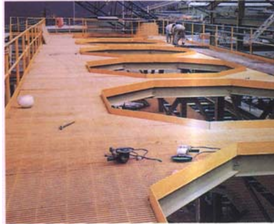
Pacific Composites' Safetread grating installed in a corrosive environment at the Porgera Gold Mine in Papua New Guinea.
